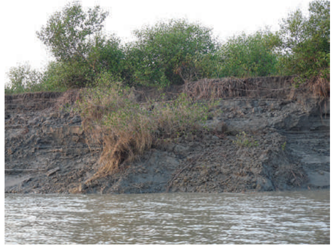
Crumbling shore as a result of highly dynamic system
