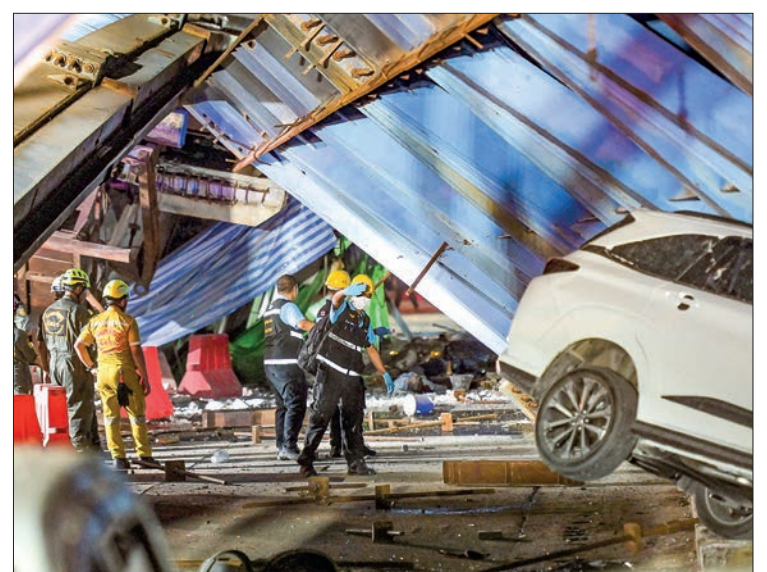
Forensic police and rescue workers inspect the scene after a construction girder on an elevated tollway collapsed, killing at least one person, in Lat Krabang district in Bangkok on 10 July 2023. PHOTO: AFP
