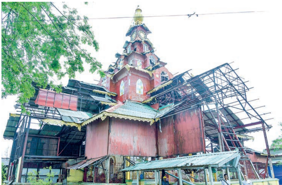
The photo shows the damage to U Ye Kyaw Thu monastery in Sittway.
