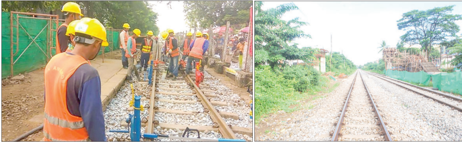
MR staff are seen working for the Yangon circular railway upgrading project.
