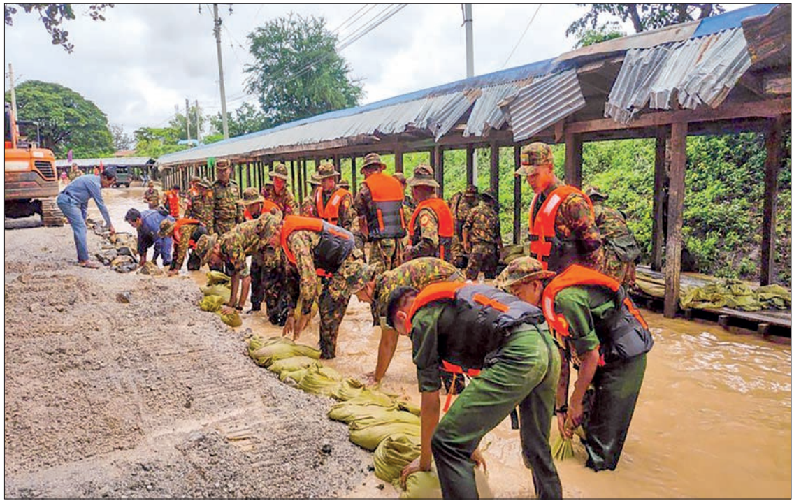
The post-flood cleanup measures underway yesterday in Nay Pyi Taw Council Area.
