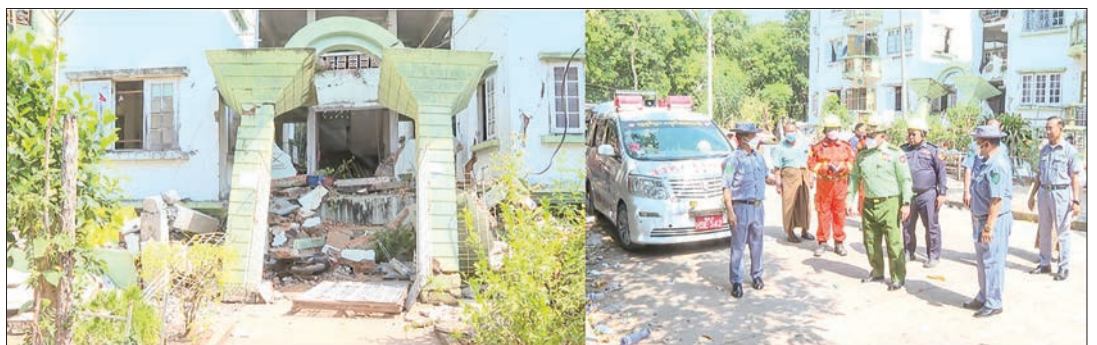
SAC Member Union Minister Lt-Gen Yar Pyae views the loss and damage at the MoBA and staff housing.
