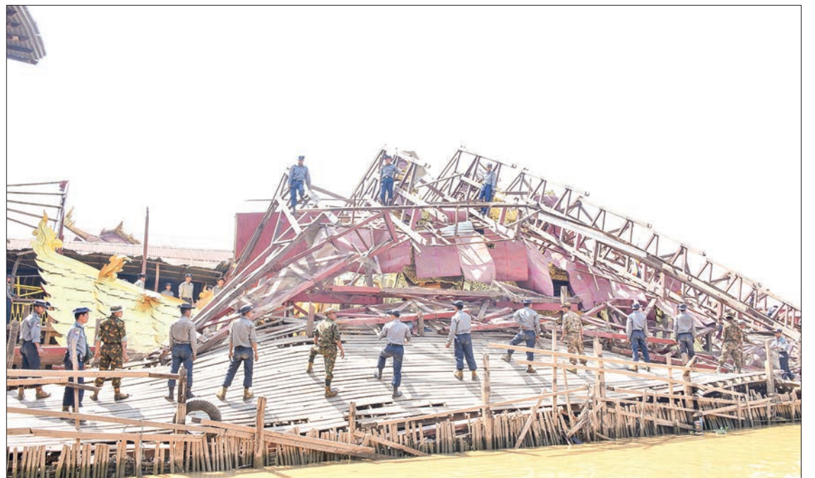
The Vice-Senior General views round the damaged structures.
